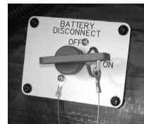
Battery Disconnect Switches
