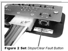
Figure 2 Set Stops/Clear Fault Button
